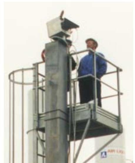
Line scanner in protective Environmental Enclosure is mounted on top of a tower.
